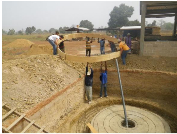
Figure 32: Lowering the outer form over the center-pole and around the rebar reinforcement
