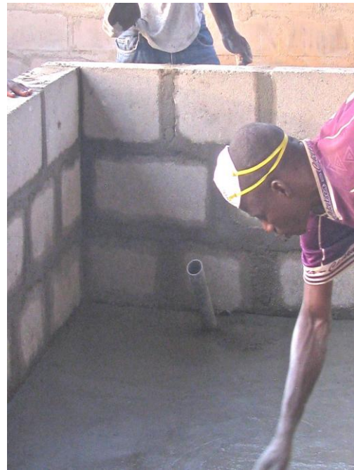
Figure 57: Outlet Detail – Grey drainage pipe (cap off) is also removable so that sludge from very bottom of tank can be cleaned out.
