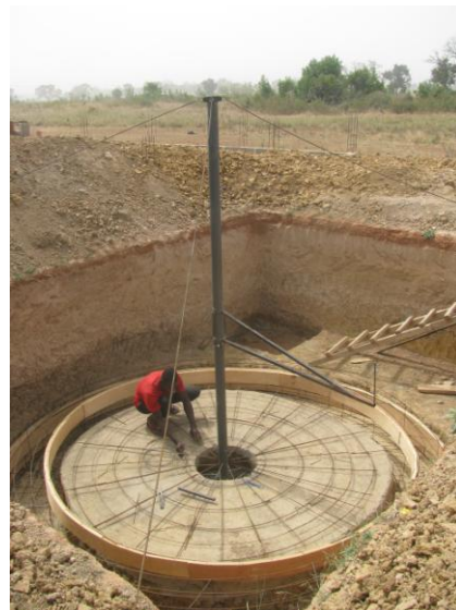
Figure 38: Roof support pole raised and centered. The steel bender continues work on rebar reinforcement
