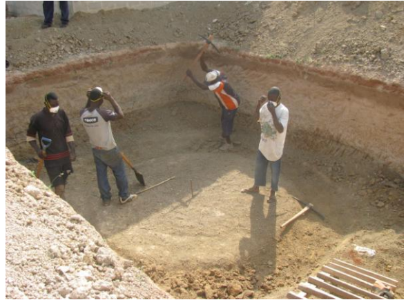
Figure 15: Using pic-axes to break up the ground and dig the tank footing
