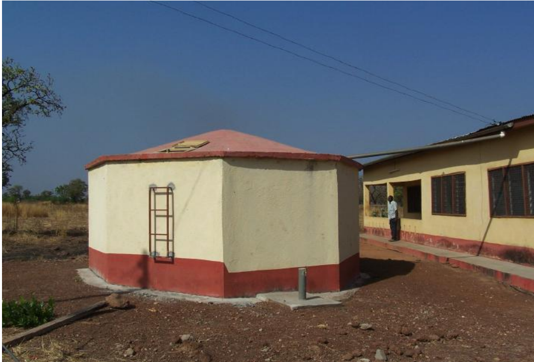
Figure 6: 30m 3 Cement Block Tank, Tamale Ghana. Red area is the approximate height of dead storage due to tap/outlet location. (Barnes 2009)
