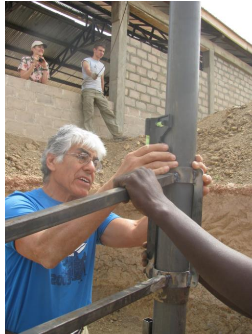
Figure 36: Securing and positioning pole exactly at tank center using a level and 4 cables
