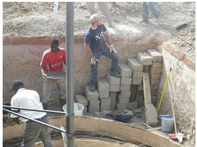
Figure 42: Foundation pouring happens one head-pan at a time. Westwood stands on the stairs ready to pass down another head-pan full of cement to Sadat, who passes to Mr. Kuma, to pour into the foundation
