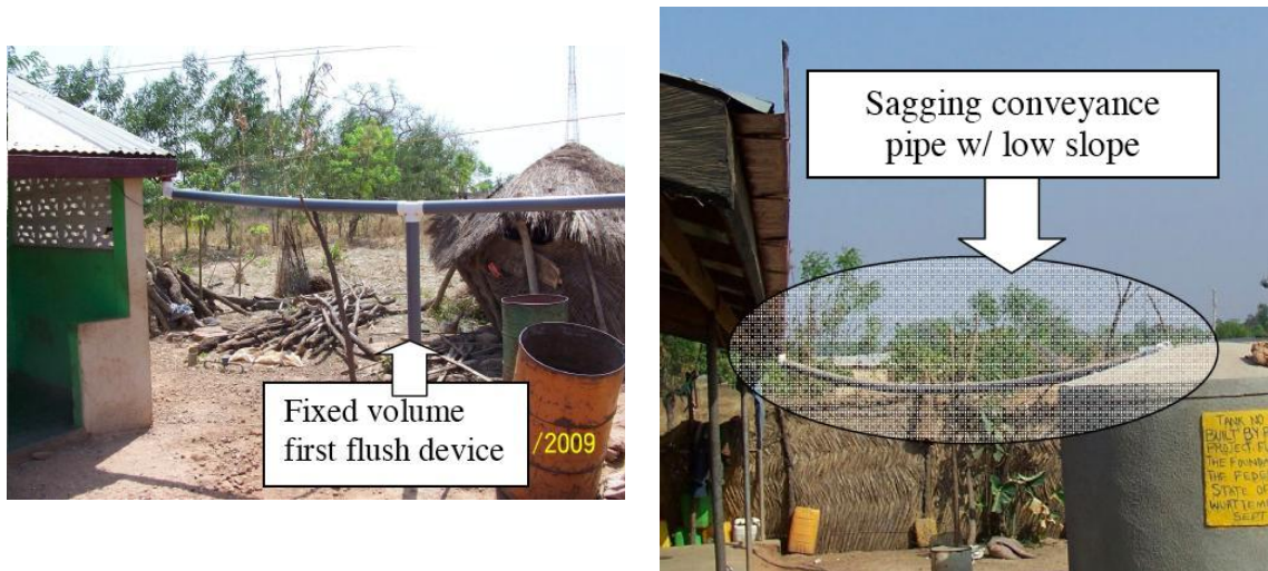
Figure 5: Fixed Volume Device (Left), Sagging Conveyance (Right) (Barnes 2009)
