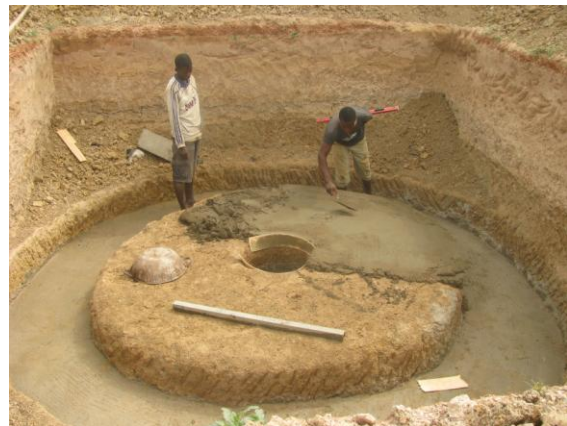
Figure 17: The mason applies a 2-inch base layer (1:3 cement to sand ratio) to the bottom of the footing, tank base
