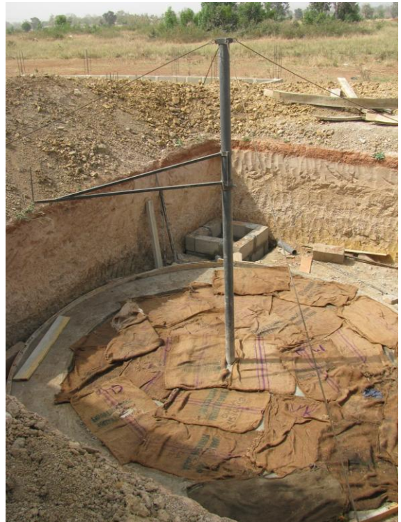
Figure 46: Finished foundation is covered with wet burlap sacks to keep it moist while concrete dries
