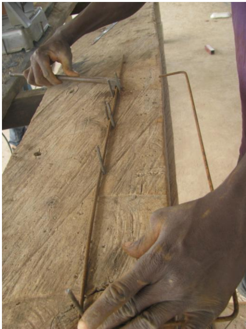
Figure 22: Close up of the jig used by the steel bender to bend rebar rod
