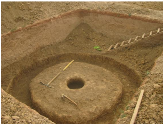
Figure 16: Footing and center hole dug and ready for 2-inch base layer center pole hole.
