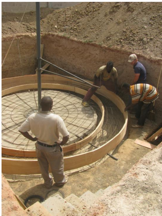
Figure 37: Using rotating arm on the center pole to ensure accurate placement of the inner form. Cutting a hole in the outer form for the placement of a 4 inch PVC outlet and drainage pipe
